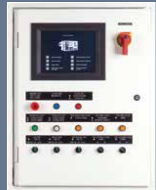
Digital Control System
